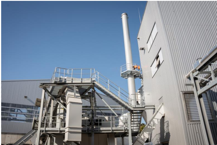
Biomass heating plant
